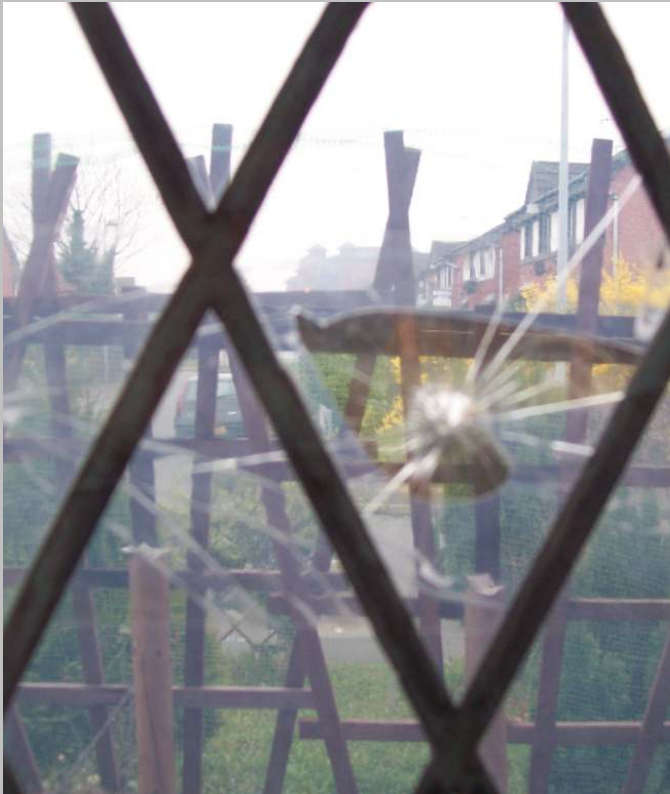
A broken window at the home of one of our members. But examples of harassment aren't always this overt.
